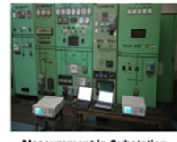
Measurement in Substation
